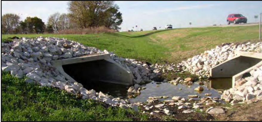
The presence of a parallel abandoned railroad compounded drainage issues by limiting the number of suitable drainage outlets.
